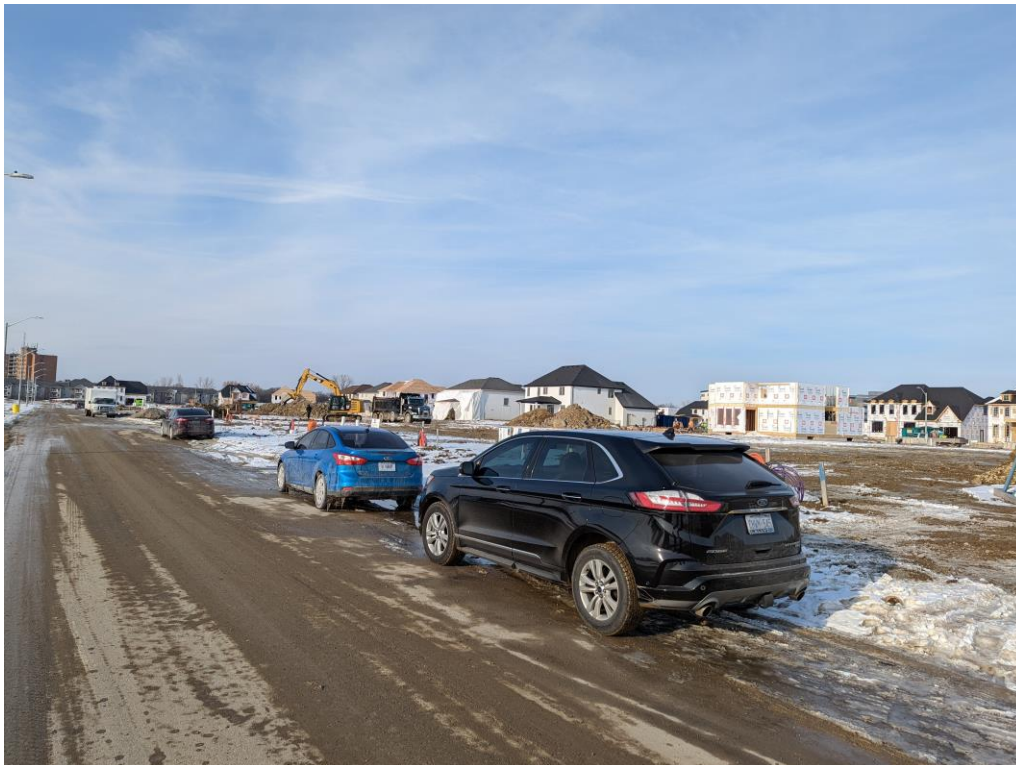
Single Unit dwellings under construction Bowler Drive, North of Spitfires Way, Looking North
